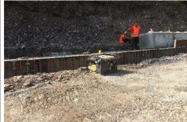
Power generator without drip tray, workers without PPE
